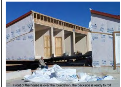
Front of the house is over the foundation, the backside is ready to roll Home is rolled onto foundation
